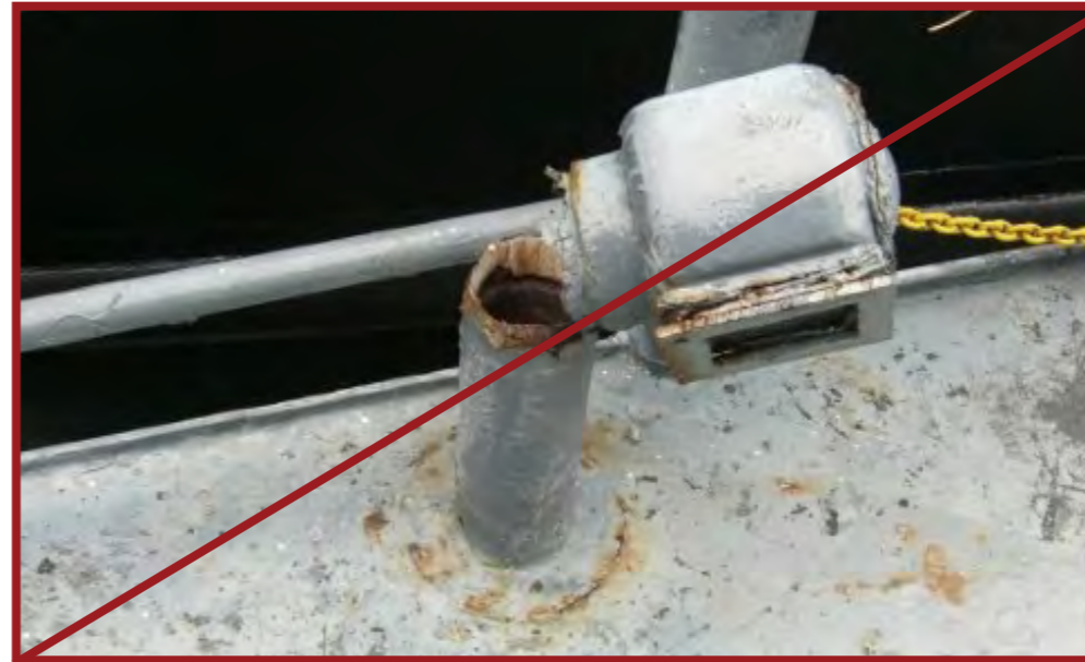
Broken vent pipe that will not pass inspection
