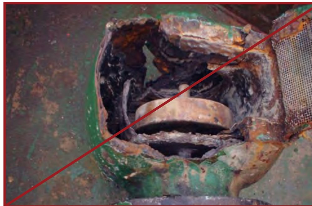
Vent head that will not pass inspection
