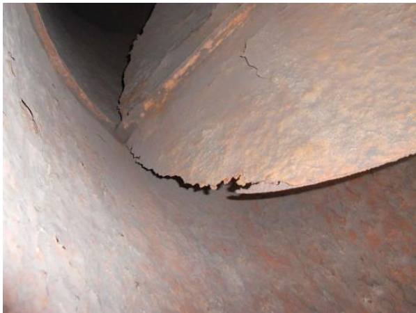
Fire damper flap wasted.
