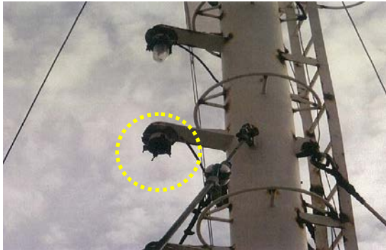
Signal light missing.
