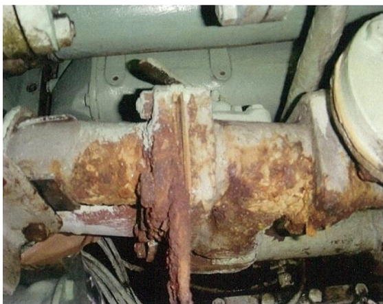
Badly corroded and leaking piping.
