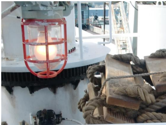
Emergency lighting at embarkation station in good condition.
