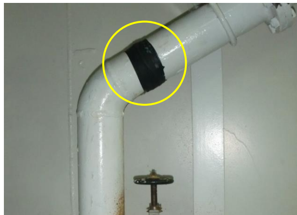
Pipe temporarily repaired with rubber patch.
