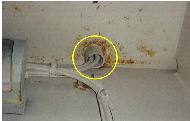
Missing sealing material of cable penetration through deck.
