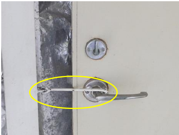
Unacceptable hold-back hook.
