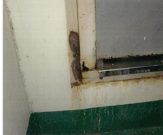
Worn-out and partially wasted fire door frame.
