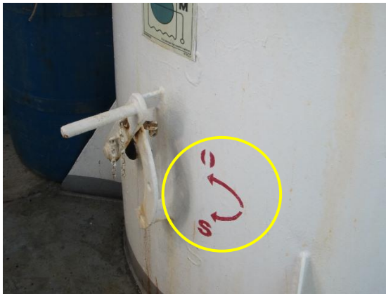
"Open-shut" positions clearly marked on ventilation trunk.
