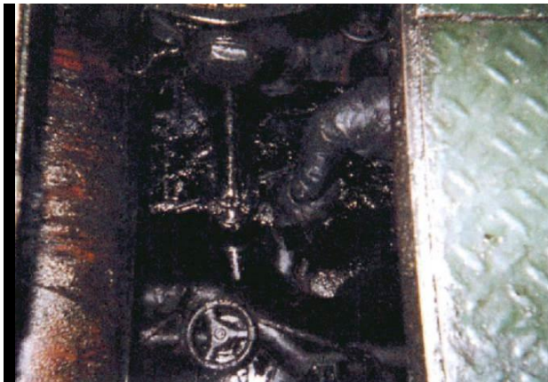
Tank top of engine room oily.
