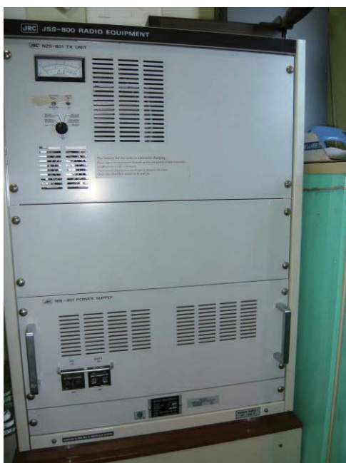
Switch Panel for MF/HF radio
