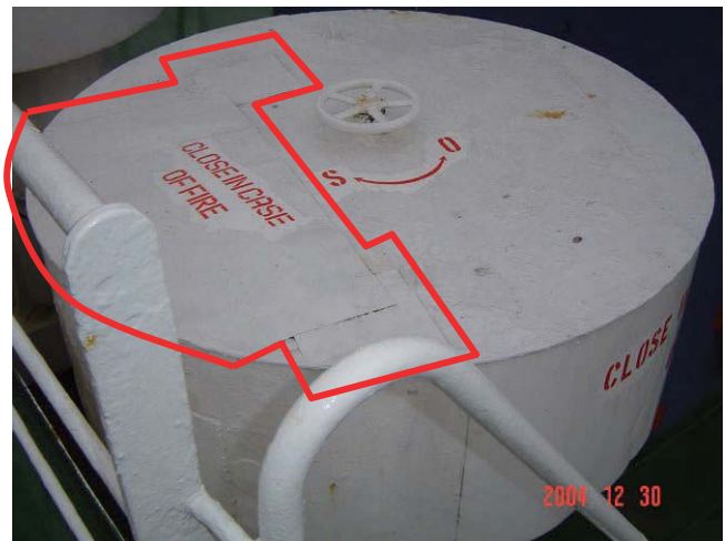
Inappropriate temporary repair by tape
