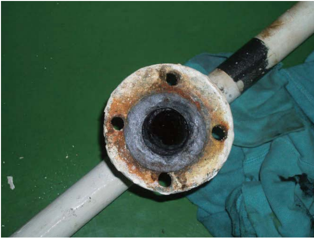
Oily inside of discharge pipe
