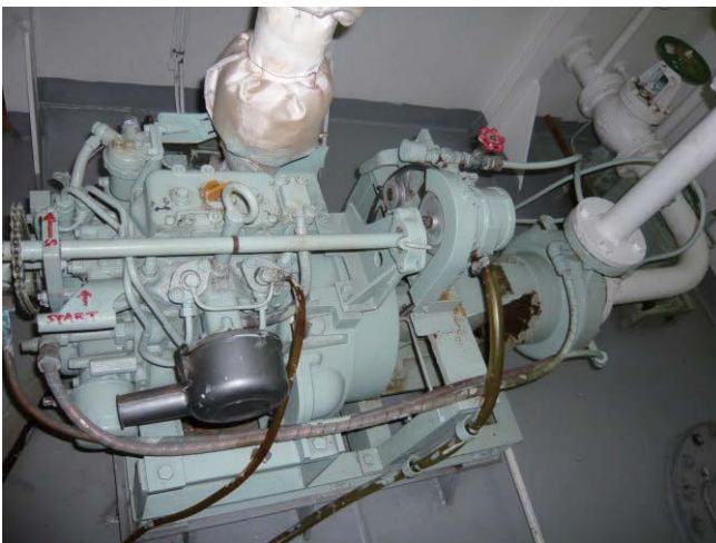
Emergency fire pump
