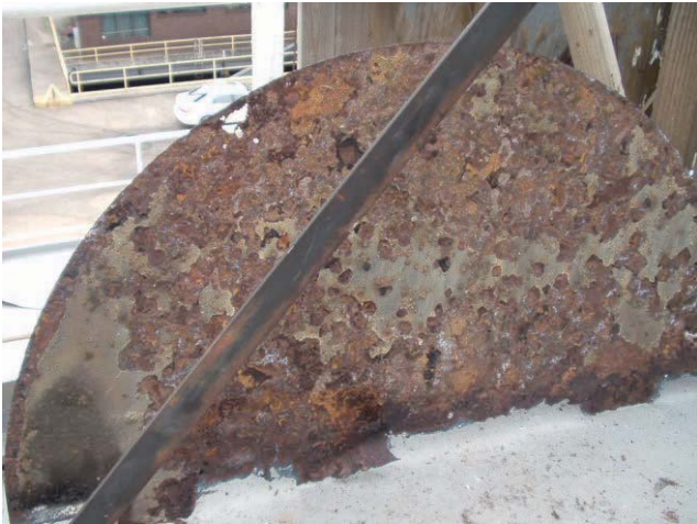
Wastage/Corrosion holes in fire damper flap
