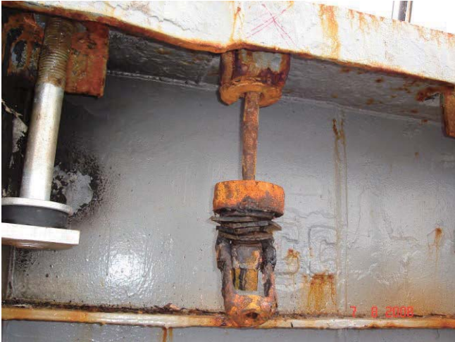
Wasted securing device
