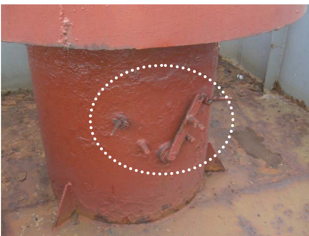
No marking of “Open-Shut”
