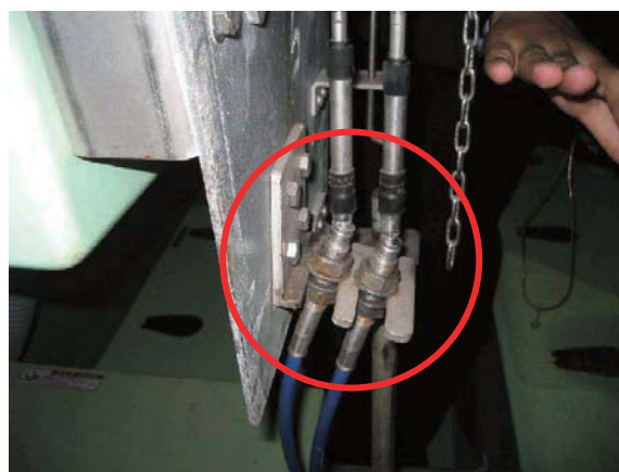
Bent release cable and bracket
