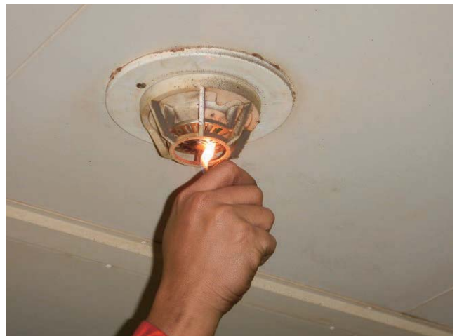
Inadequate test method
