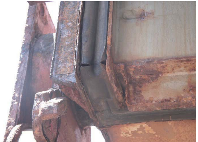
Deteriorated and cracked rubber packing
