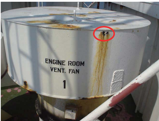
Corrosion holes in the casing of ventilator
