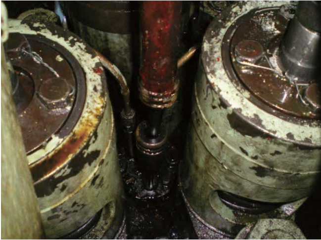
Partial lack of a high-pressure fuel oil pipe doubling jacket
