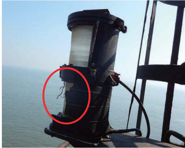
Damaged navigation light
