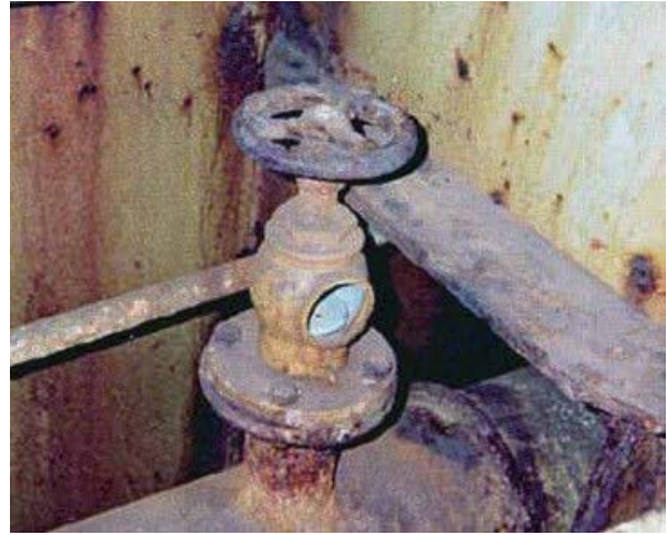
Missing of coupling
