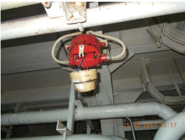
Defective of fire detector
