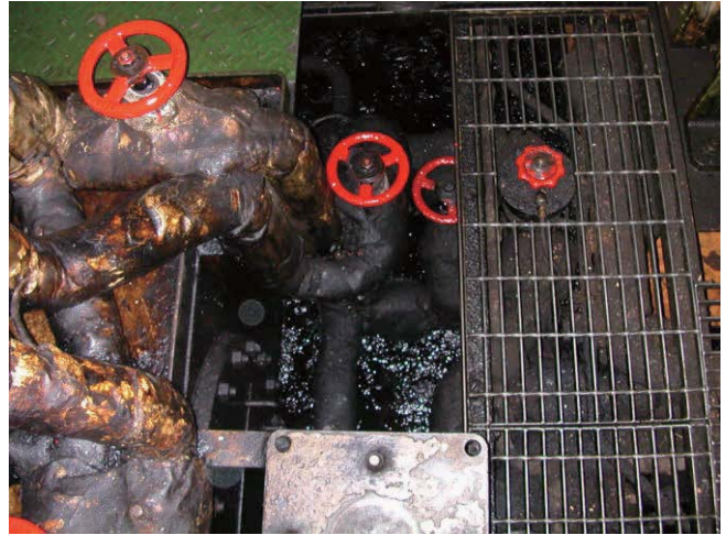
Dirty Engine room tank top
