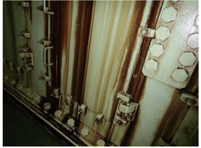
Oil leakage of M/E
