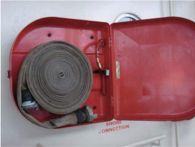
Missing of fire nozzle
