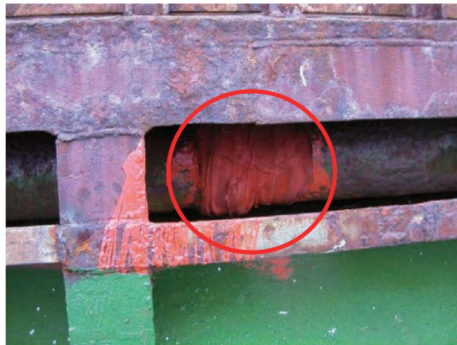
Inappropriate repair by cloth
