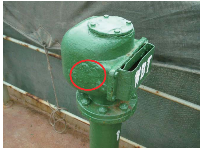
Inappropriate temporary repaired by putty
