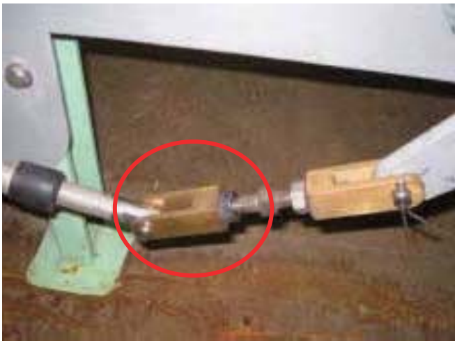
Incorrect condition of turn buckle
