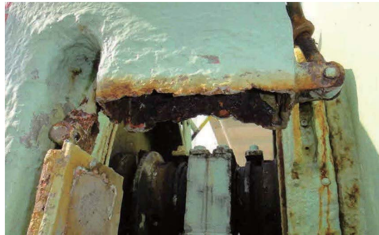
Wasted gooseneck ventilator
