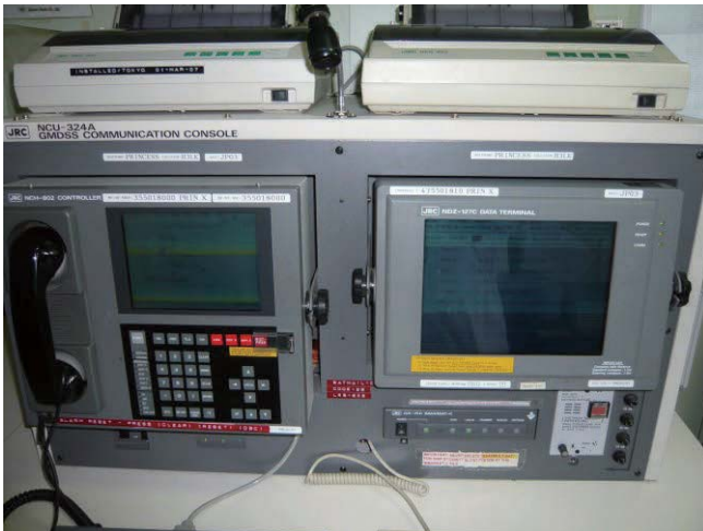
GMDSS communication console
