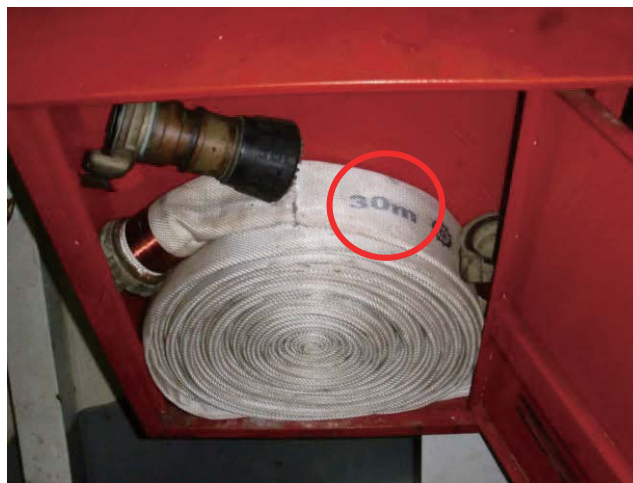
Length of fire hoses in E/R is not to be more than 15m
