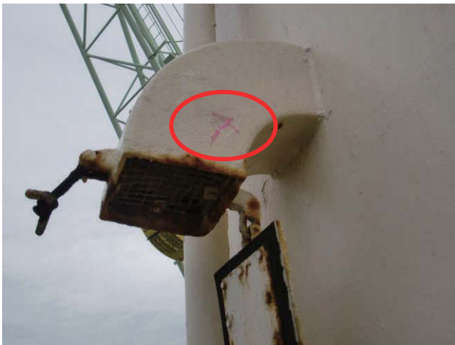
Hole with inappropriate repair with tapes
