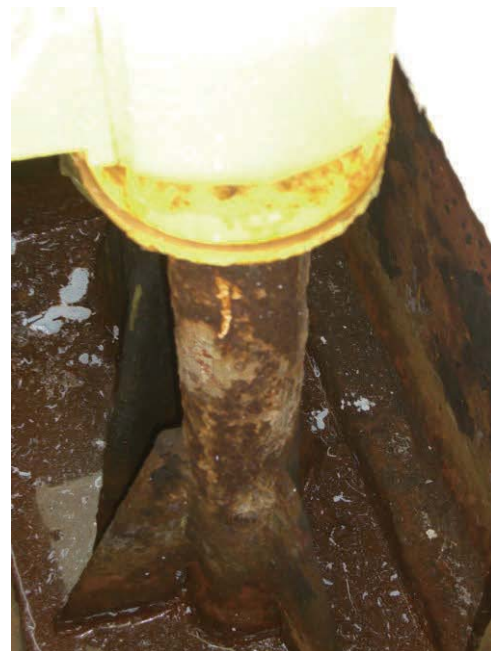
Wastage of air pipe
