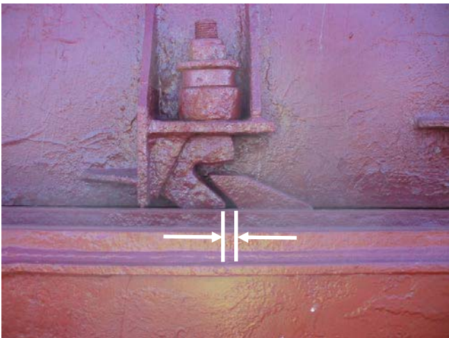
Excessive gap of hatch cover side cleat
