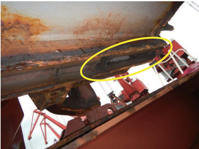
Partly missing rubber packing
