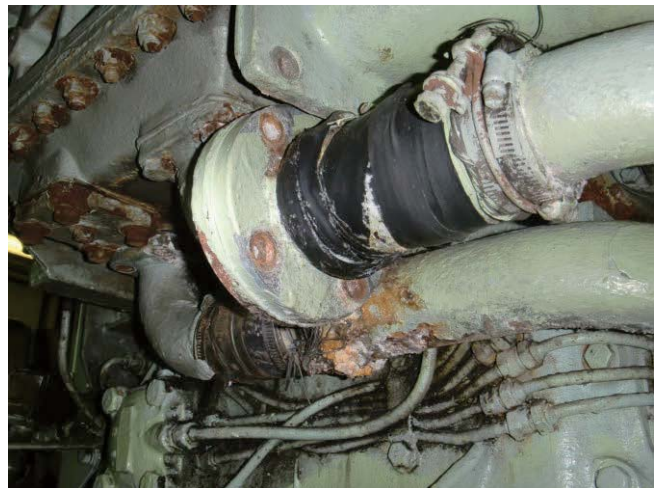
Inappropriate repairs by rubber patch on SW pipe for G/E
