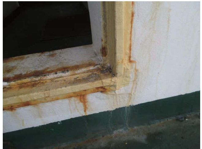
Wastage of door frame
