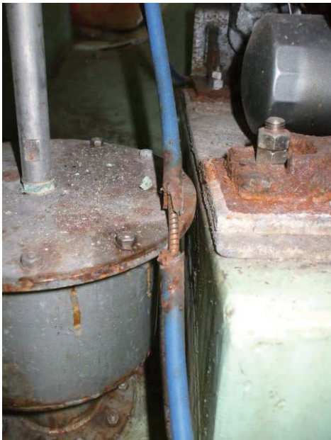
Defective release cable
