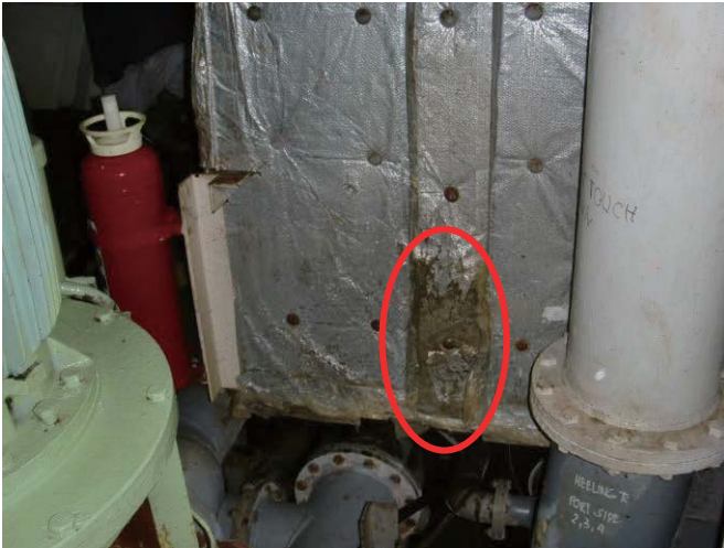
Partly missing A-60 class insulation
