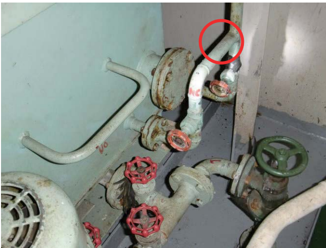
Inappropriate repairs by rubber patch and plastic putty
