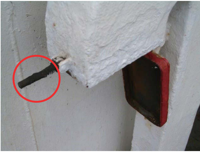
Missing butterfly nut of gooseneck ventilator
