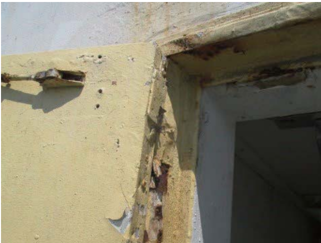
Wastage of door and door frame
