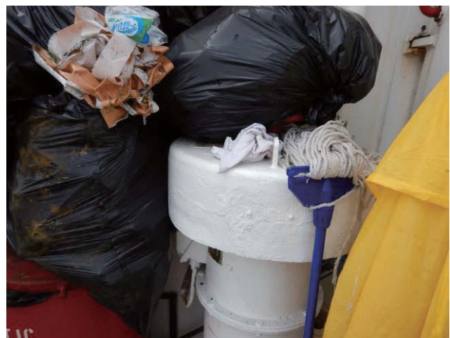
Ventilator is obstructed by garbage
