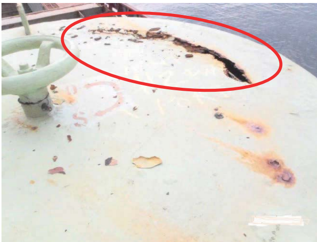
Corrosion holes in the casing of ventilator
