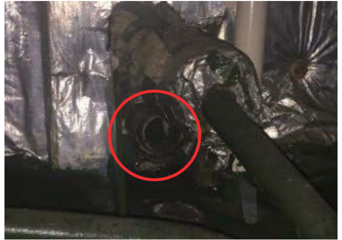
A hole on the A-60 class bulkhead
