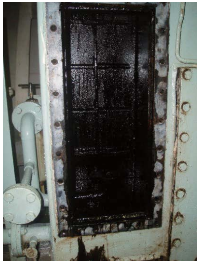
Oily inside of oil water separator
