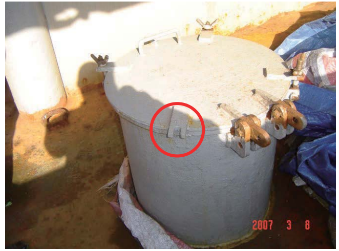
Missing nut and bracket with bolt
