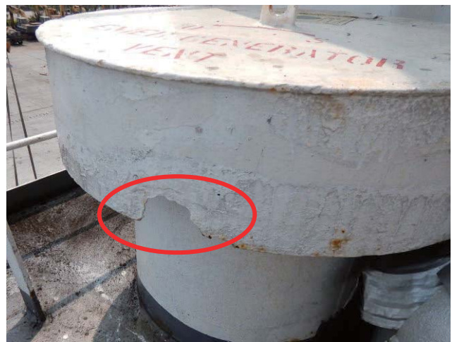
Wastage of the casing of ventilator
